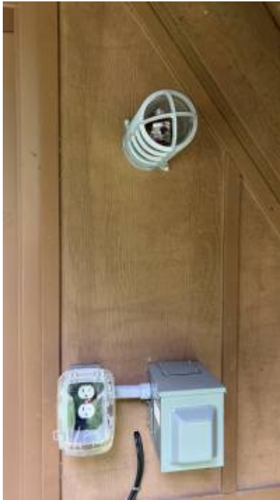
Figure 1: The pump house alarm indicator light
