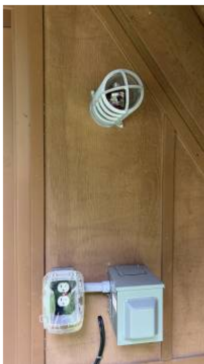
Figure 1: The pump house alarm indicator light
