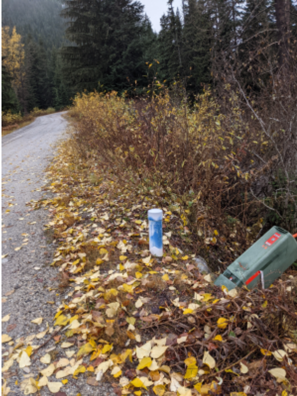
Blowoff Division Three Bottom
