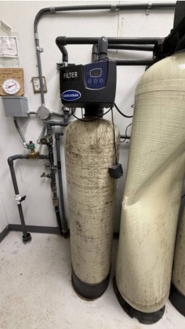
Debris Filter Tank
