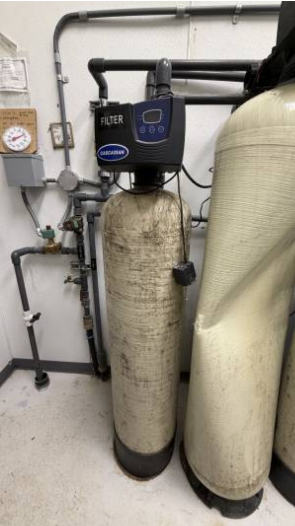
Debris Filter Tank
