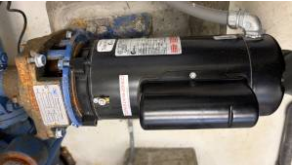
Booster Pump Right Motor
