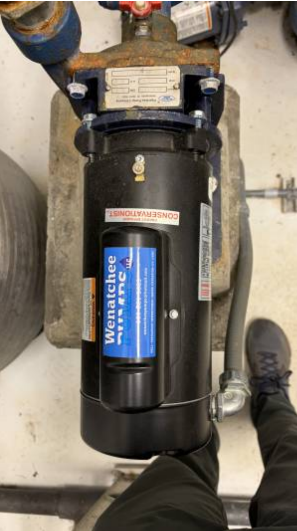
Booster Pump Left Motor
