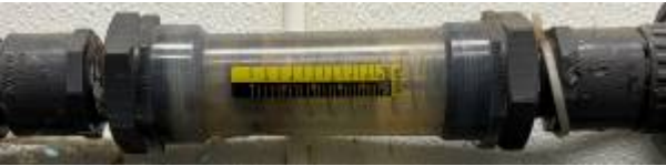
Well Flow Meter
